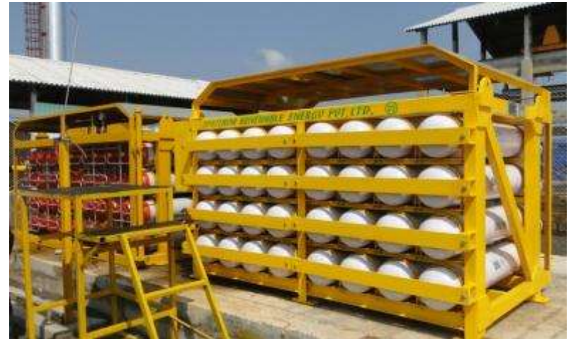
Bio-CNG Filled Cascades
